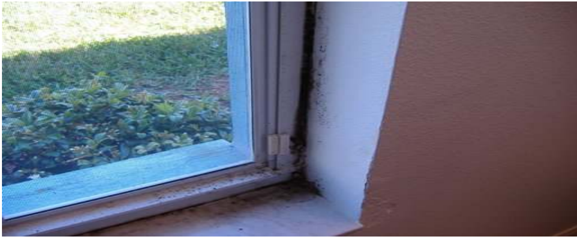
Photo 5 - Below, mold is growing on the bottom of the doors.
