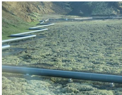
Pipes carrying the hot water
